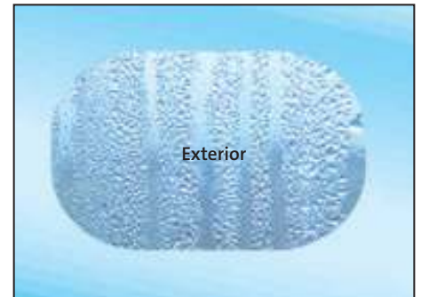
Condensation on the exterior face of a DGU.
